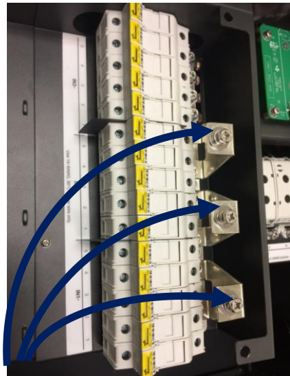
Figure 9-4 Bypass Terminals Installed on NEG Bus
