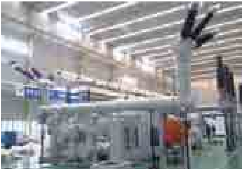
Kiev Boryspil International Airport-126kV GIS The Ukrainian Kiev Boryspil International Airport Project is one of the important projects from the 2012 European Cup.
